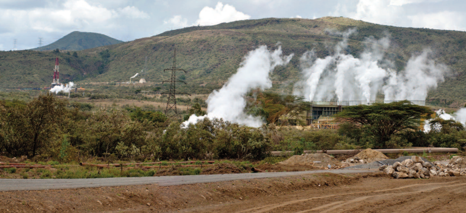
Olkaria II geothermal power plant – iStock, Byelikova Oksana
